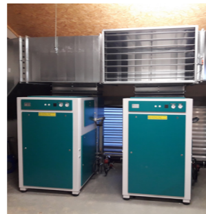
Compressor with venting system
