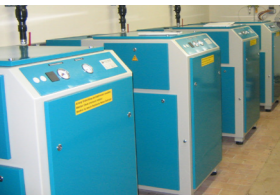
Compressors in the plant room
