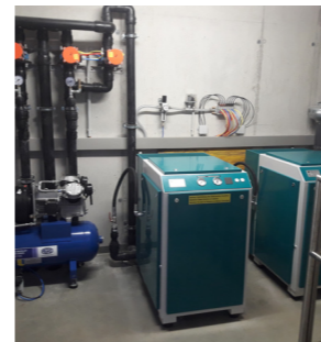
Compressor with process air flow
