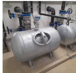
Collecting vessel with piping
