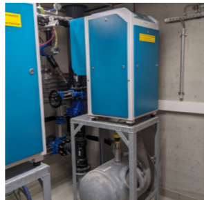
Machinery room with compressors
