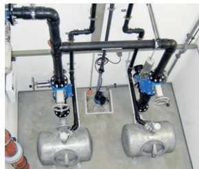
Equipment in a pump room
