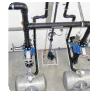
Equipment in a pump room
