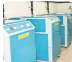
Compressors in the plant room
